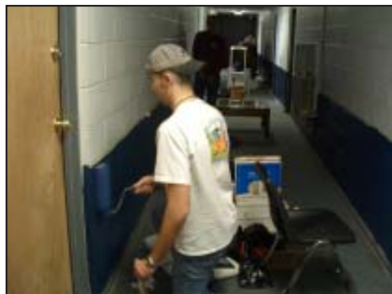
Brother Ryan Hannebaum puts a new coating of paint on the walls on the third floor of the Chapter House.
